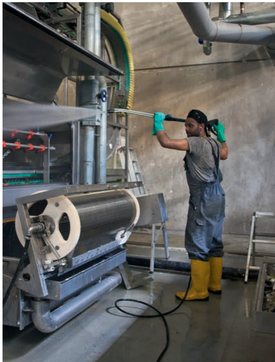
Washing plant for returnable carriers
